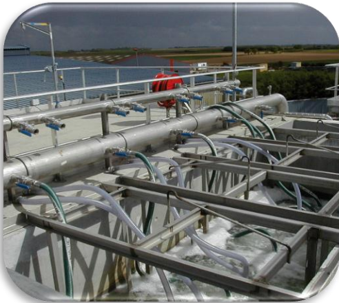
MBR Membrane Bio Reactor
