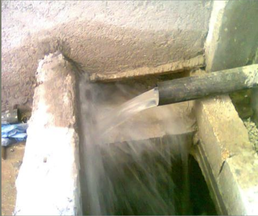
Effluent stream of the aeration process
