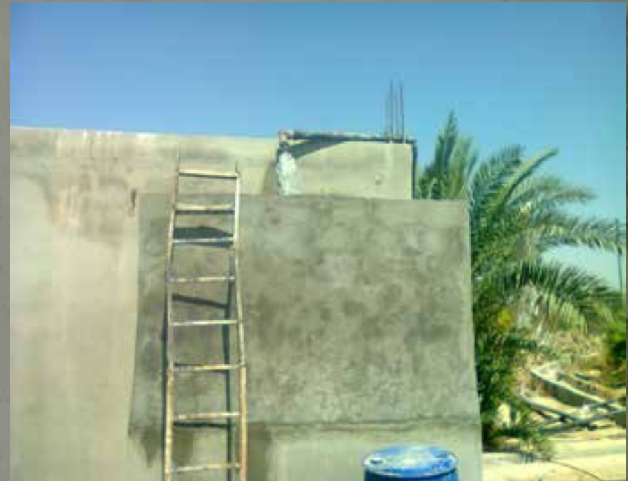
Side view of the free fall Aeration
