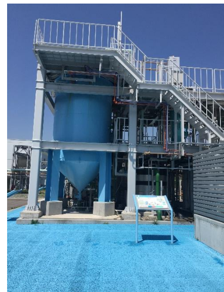
Phosphorus Recovery Unit
