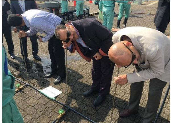
Mission team members try to hear the noise of the leak
