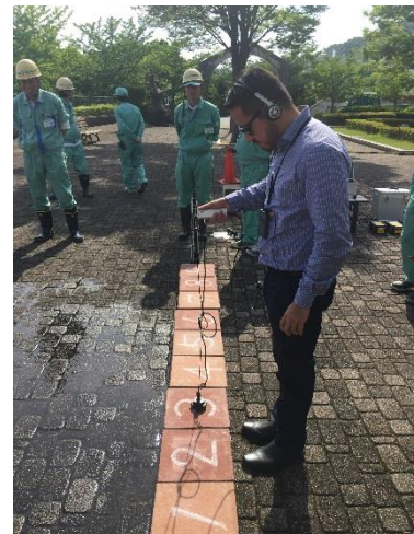
Mr. Villegas Lira tries to find the leak point using electronic acoustic bar
