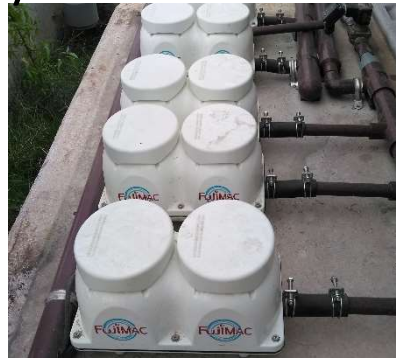
Only Small blowers need electricity
