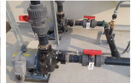
Many devices need electricity
