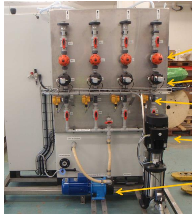
SVP-Pure ® ClO 2 generator + four-point dosing system
