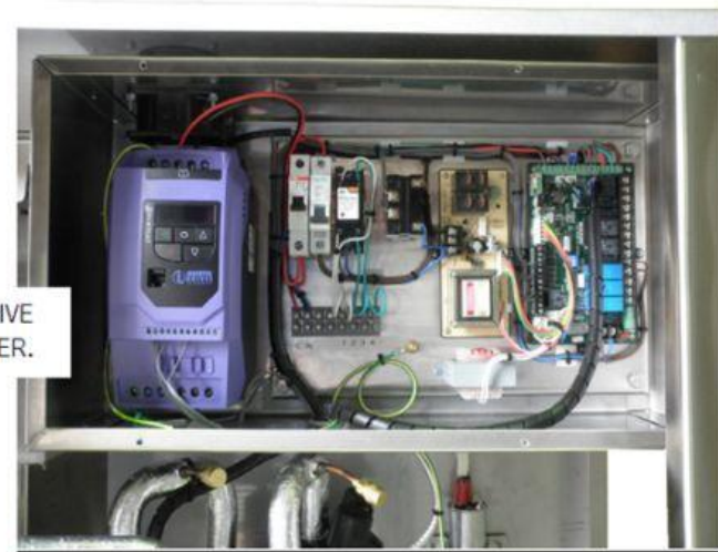
Electrical panel with cover removed.
