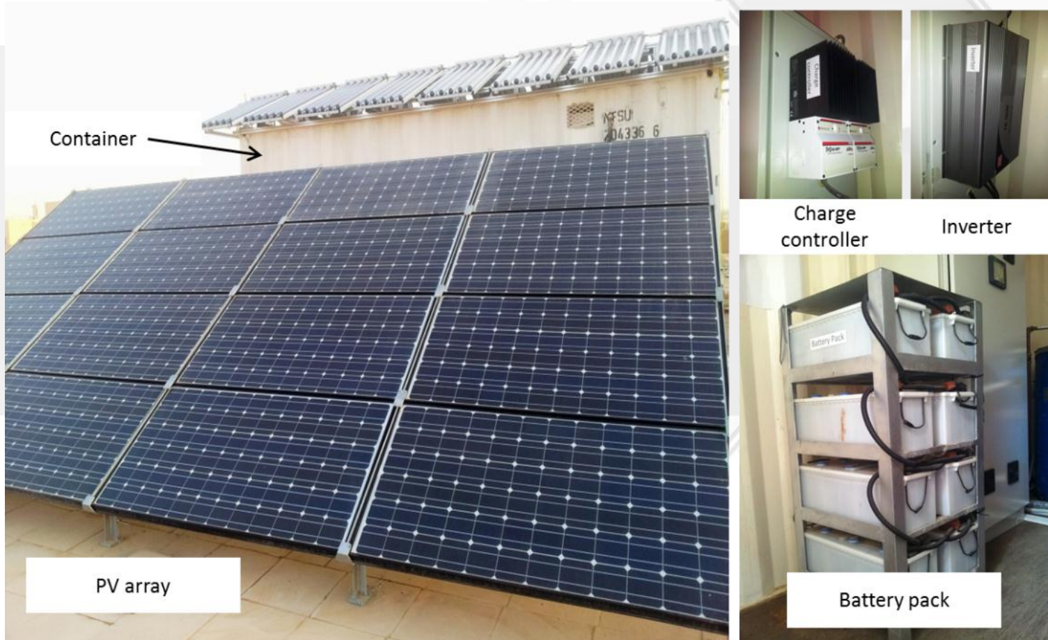
Figure 16. Photograph of the PV array beside the container
